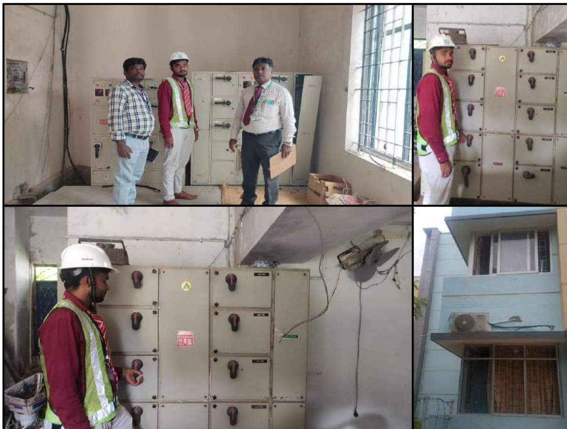
Energy conservation facilities observed in the Campus
