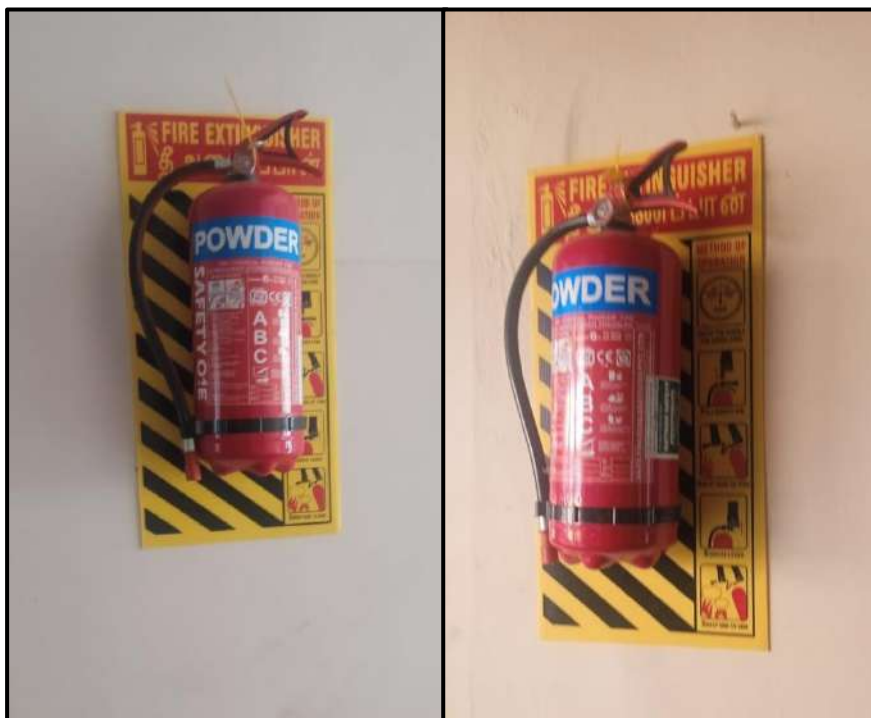
Fire Extinguishers designed at the campus to ensure the safety of the Stakeholders
