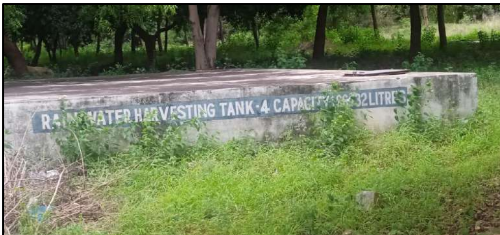
Rainwater Harvesting units observed in the organization
